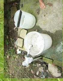
Tap receiving water from groundwater works
